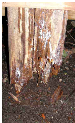
Deteriorated post in direct contact with soil.
