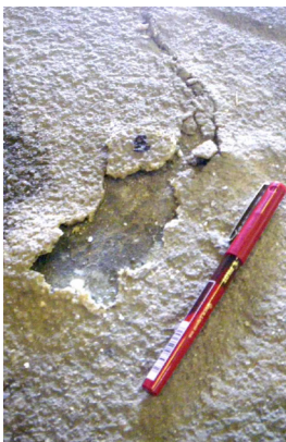
Delamination of suspended concrete slab membrane
