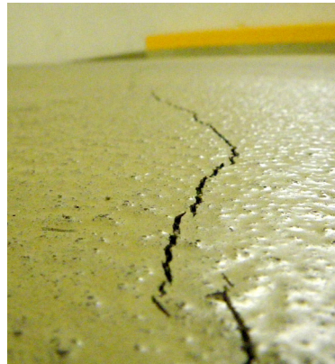
Cracks in a suspended concrete slab membrane
