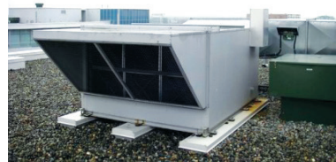
Typical rooftop make-up air unit
