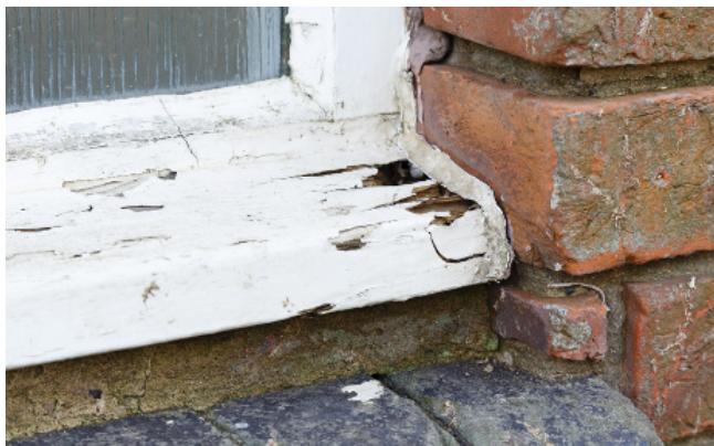
A rotten wood frame window
