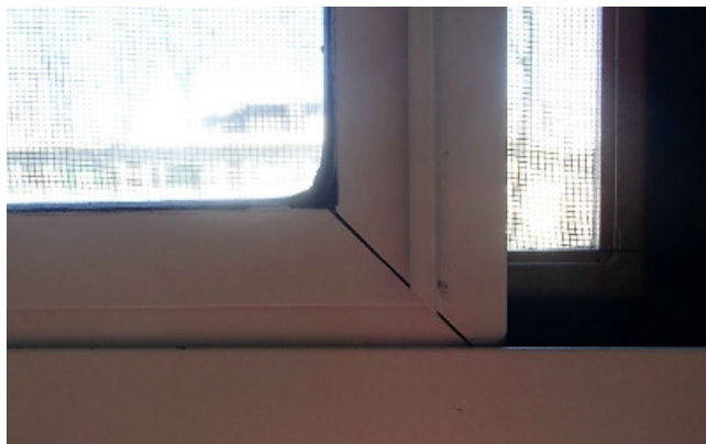
Misaligned miter at the corner of aluminum window frame
