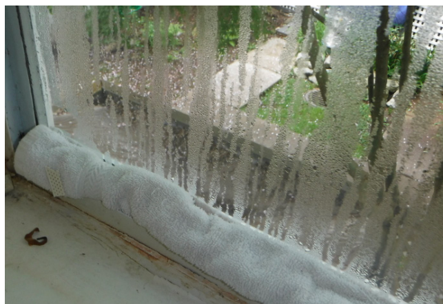
Condensation on the interior of the glass
