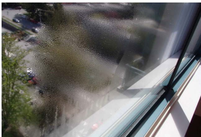
Fogged, failed IGU
