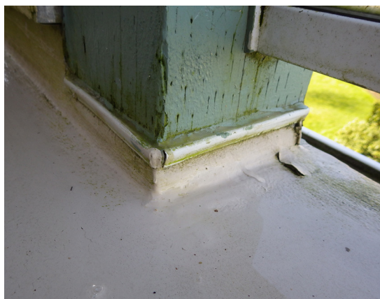
Figure 4 – Failure of the balcony membrane
