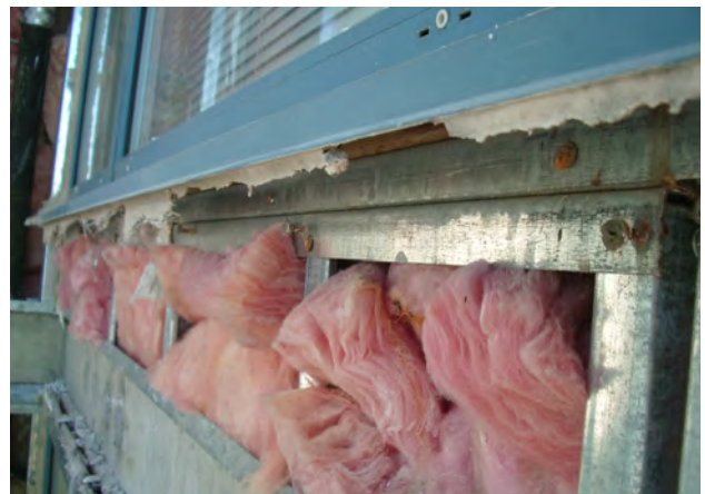
Corroded screws in stud wall beneath window
