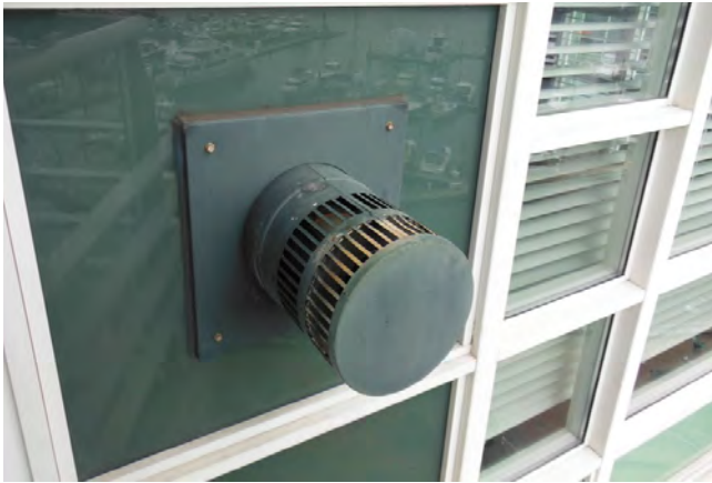
Fireplace vent penetration through a spandrel panel
