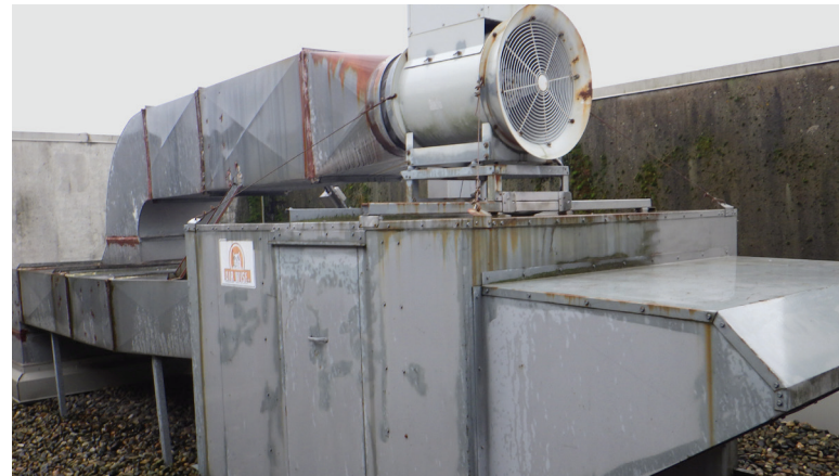
Figure 1: MUA with fire exhaust.
