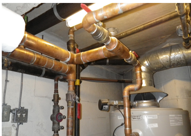
Example of uninsulated copper piping
