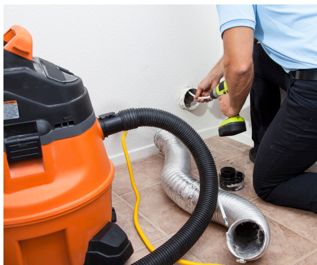
Cleaning and maintaining dryer exhaust vents
