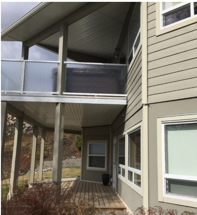
Average size hot tub placed on a second-floor, wood-framed balcony
